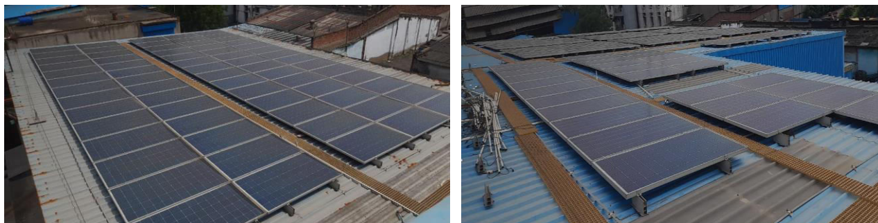
Existing solar plant of the company at Manufacturing Unit
